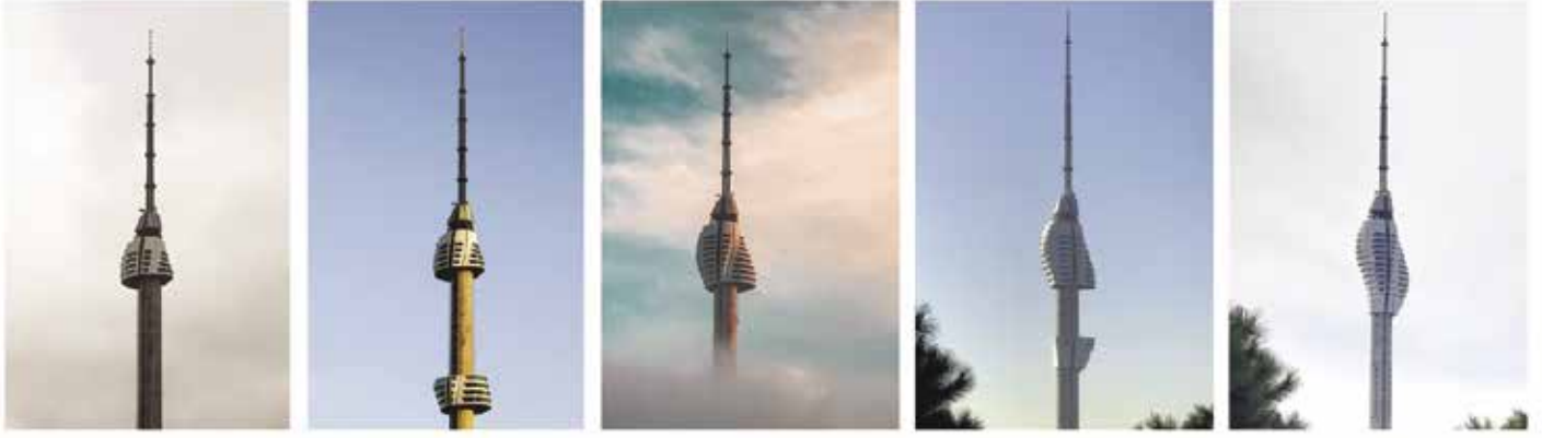
10 İstanbul TV-Radyo Kulesi inşa süreci (©MAA - MELIKE ALTINISIK ARCHITECTS). 11 Achrome[scape], 2018 (©MAA - MELIKE ALTINISIK ARCHITECTS).
